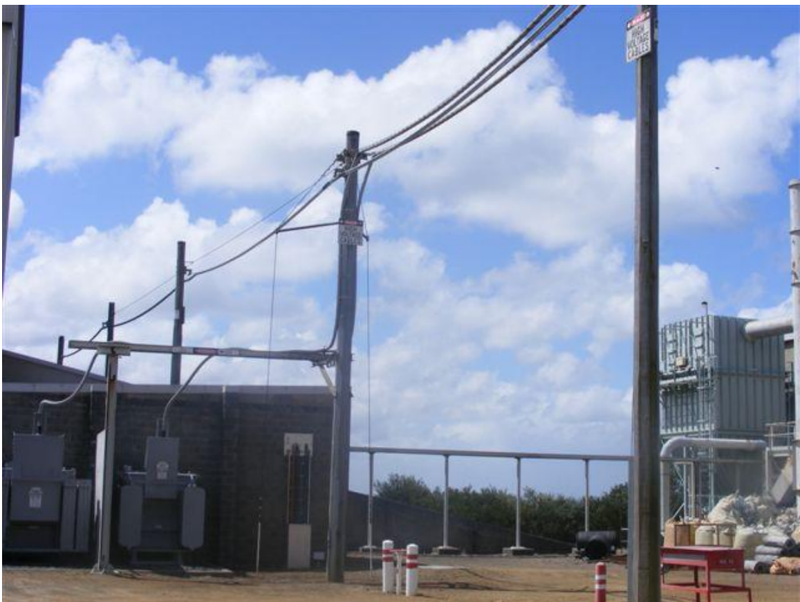
PORTLAND 22kV AERIAL LINES SHOWING THE INSULATED CABLE CONSTRUCTION AND LACK OF SIGNIFICANT VEGETATION
