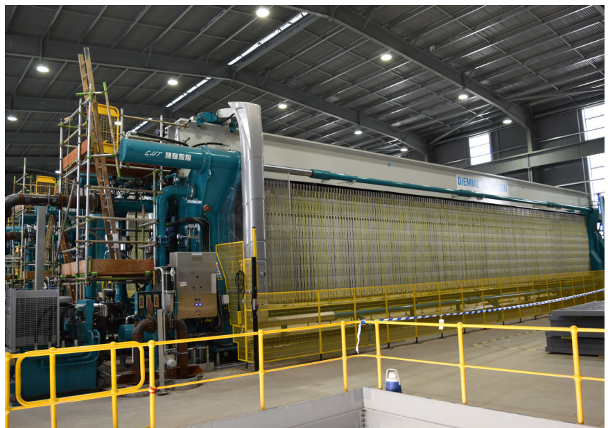
Figure A: Kwinana Refinery Residue Filtration Facility
