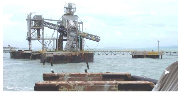
The destroyed pier seen the day after Hurricane Dean in September 2007.
