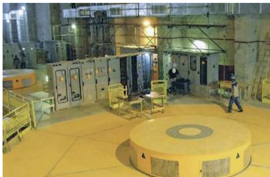
Detail of generation unit 2 of the Power House
