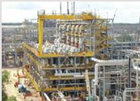
① Digestion: The goal is to promote the reaction of soda with the alumina present in the slurry (bauxite slurry), transforming it into sodium aluminate.
