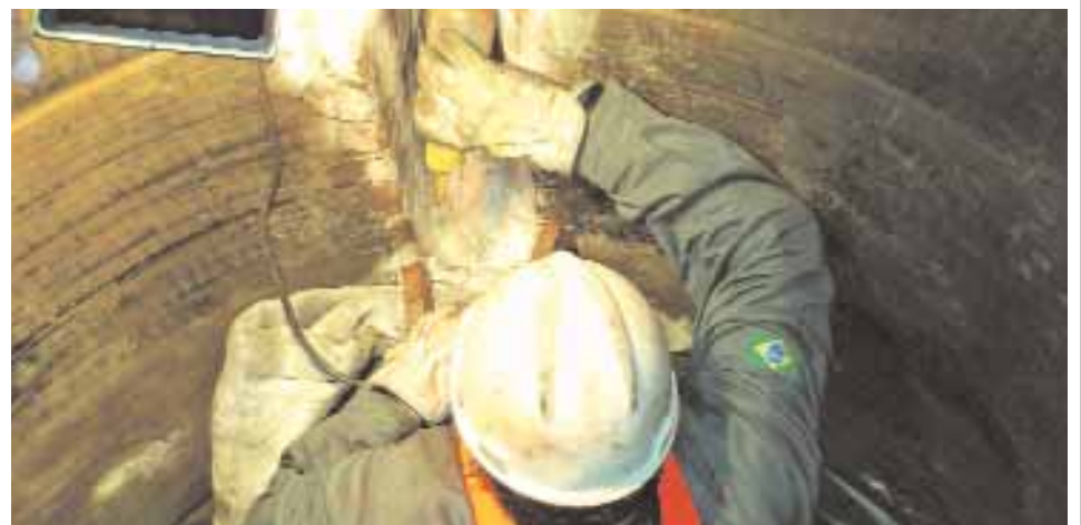
› SAFETY | Annual maintenance of 3,500 Press repaired a crack on the equipment
