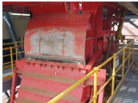
450 HOK Train Loading Bin 1
