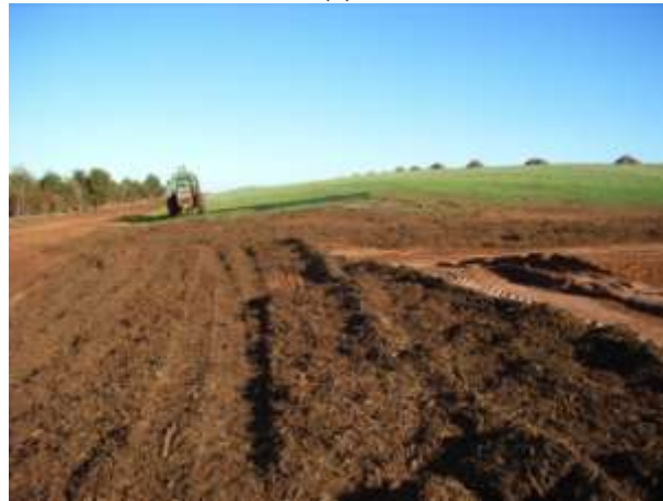
Figure 29. (a) Grading the outside area of the lysimeter facility to minimise any run-on water, (b) applying wood mulch to outside area for dust control, and (c) final wood mulch cover outside lysimeter
