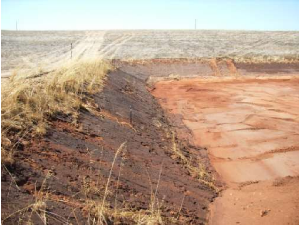
Figure 12. Western and northern boundaries were considered stable and so were not excavated for the initial 1.5 m lift
