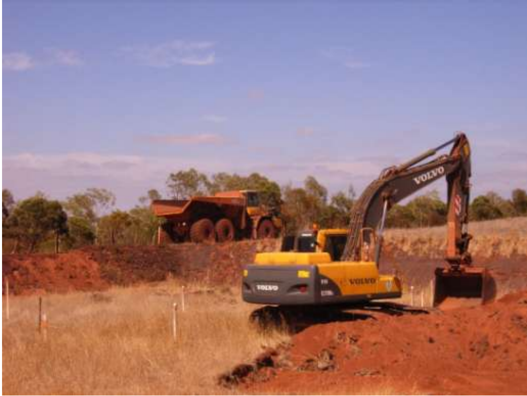
Figure 10. Clearing existing vegetation and infrastructure from Cell 4 in preparation of new lysimeter construction
