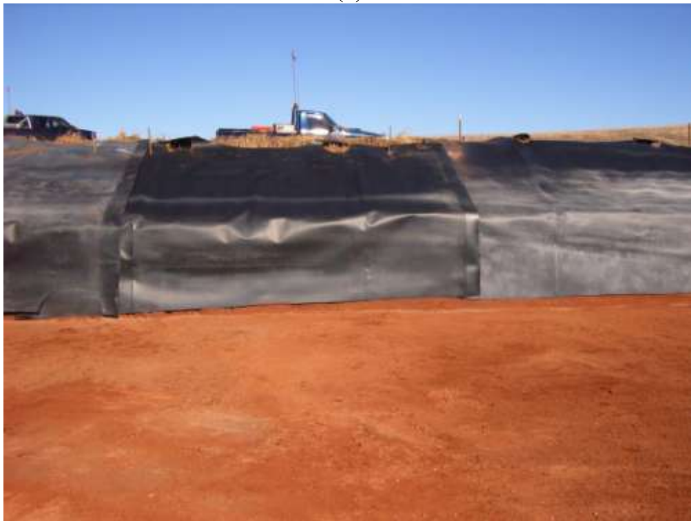
Figure 18. (a) Presence of gravel road base material in perimeter wall and (b) use of HDPE to provide a protective layer for the PVC liner prior to installation
