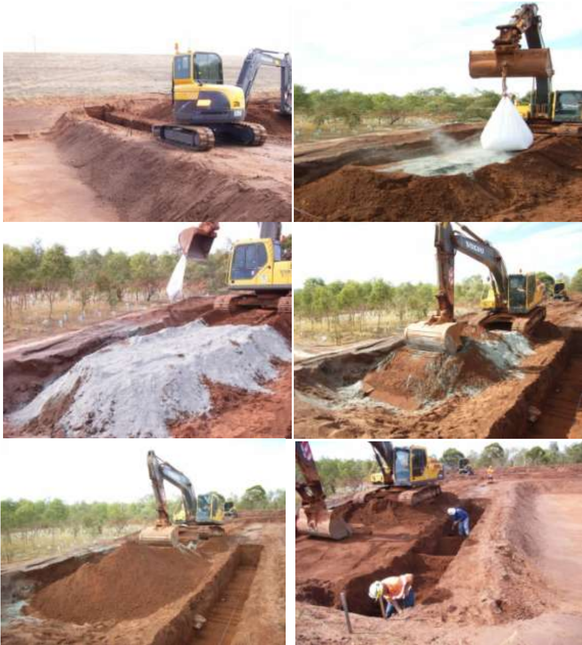
Figure 15. Mixing cement with residue sand before replacing back into trench. Once replaced the cement/sand mixture was wetted up and compacted
