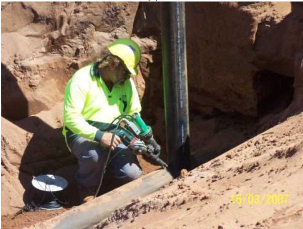
Figure 24. (a) Inspection standpipe installed into sump drain pipe, and (b) ensuring the standpipe connection is well-sealed
