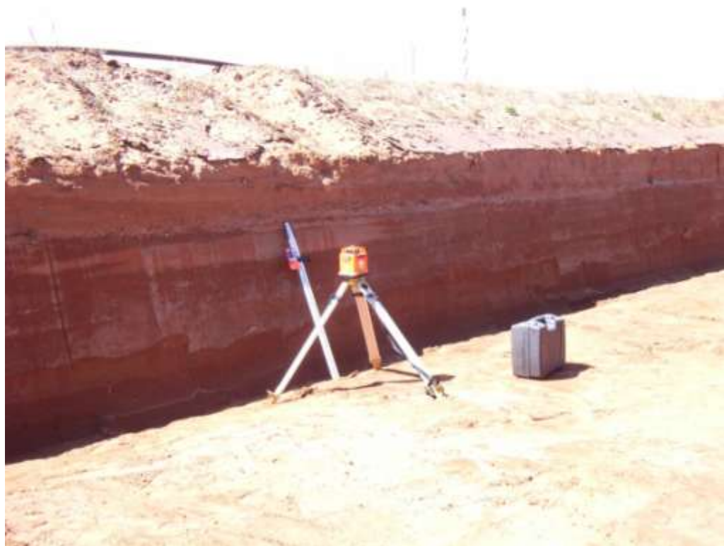
Figure 16. Removal of excess residue sand to produce a vertical wall around lysimeter perimeter
