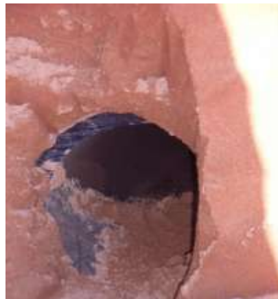
Figure 13. Pipe sleeve was installed through the eastern wall of lysimeter for sump drain exit
