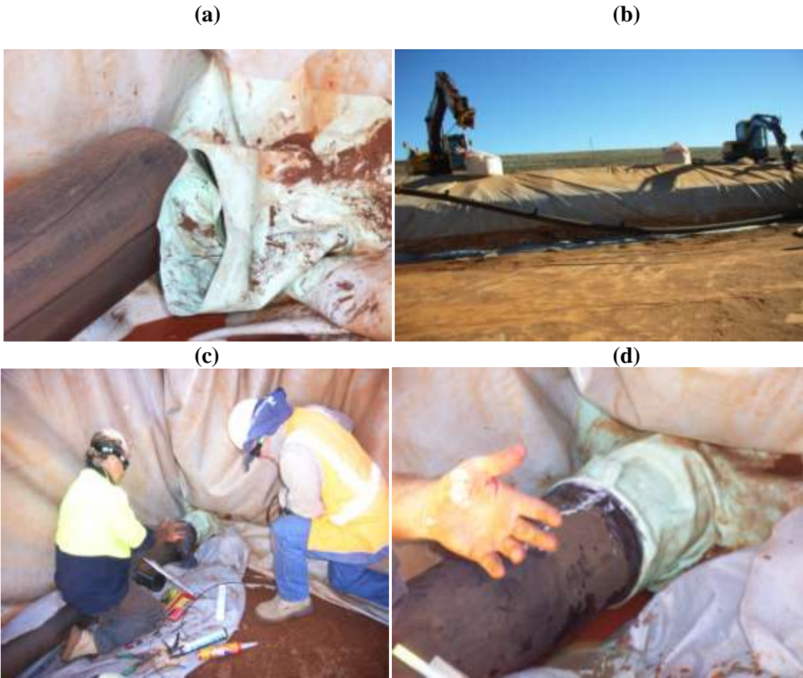
Figure 21. (a) Making a sleeve in PVC liner to allow sump drain pipe to pass through, (b) placing the sump drain pipe into the floor of the lysimeter along the northern boundary, (c) gluing the PVC sleeve around the sump drain, and (d) successful sealing of PVC liner to ensure no water loss through PVC liner
