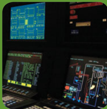
Some of the important monitoring equipment in the power station's control room.
