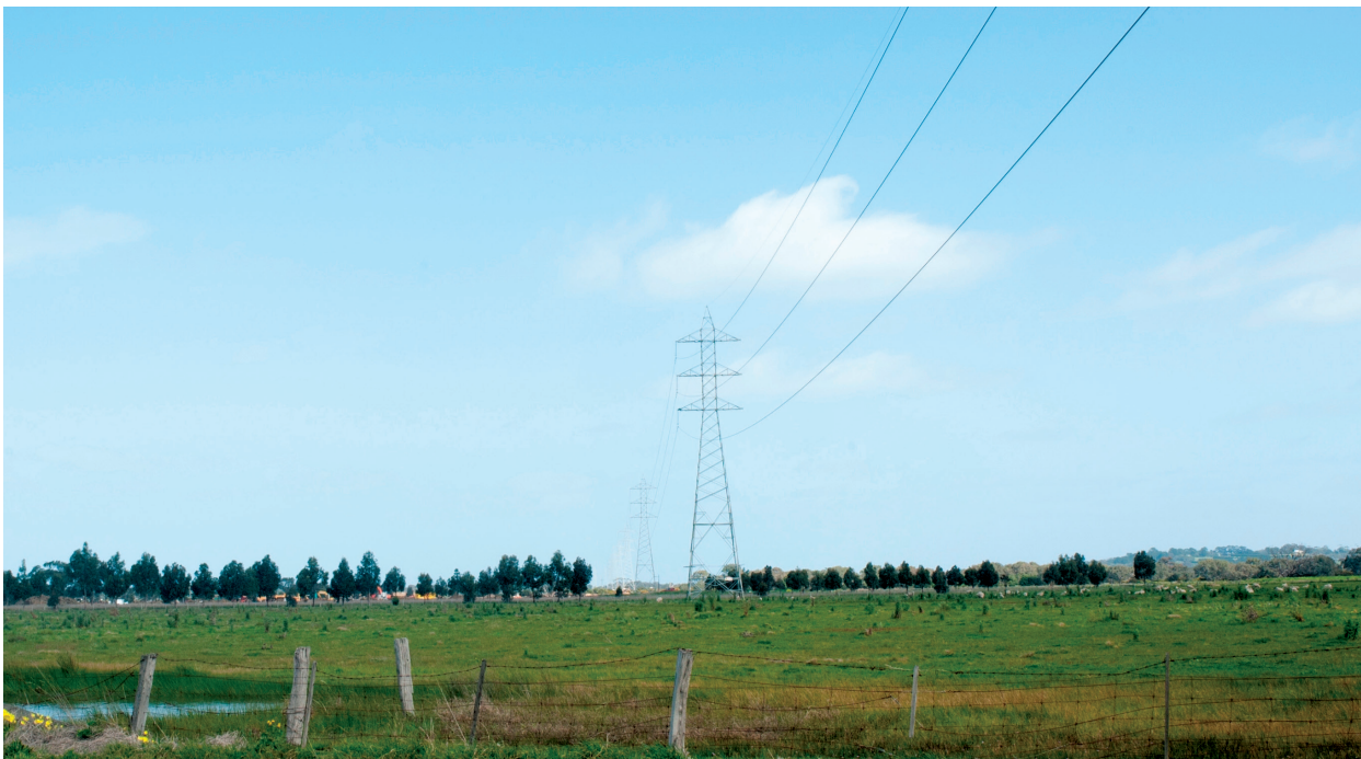
The Anglesea-Point Henry transmission line assets are to be removed.
