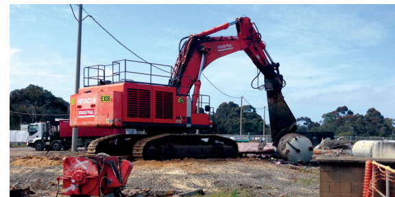
Recent decommissioning activities have included the removal of the cooling tower, workshops, tanks, water treatment plant and crushers.
