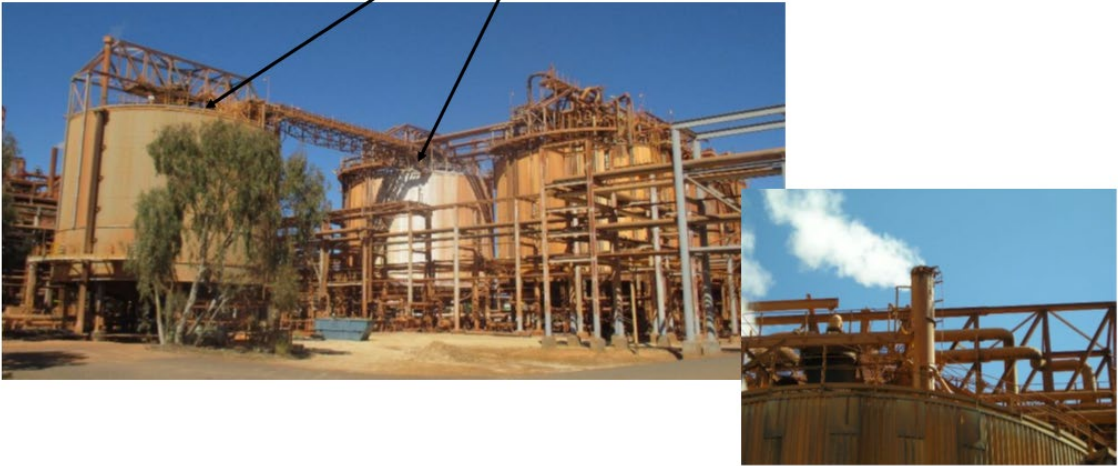
25A Tanks – Partial Treatment – 25A4 and 25A2
